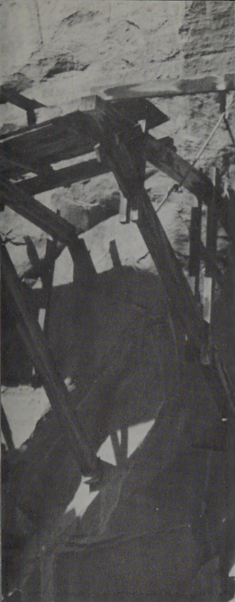
The bracing system of the flume is supported by hand-cut rock notches and blacksmithed bolts driven into the sandstone face of the Dolores Canyon walls.
